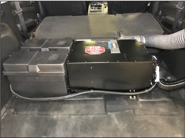
The no-idle HVAC system is installed behind the back seats of two Chevrolet Tahoes used by INL Security staff.
